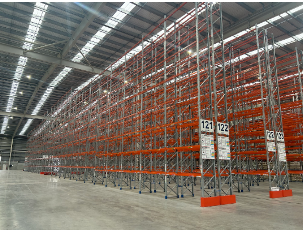
Stage 2 Racking Recently Completed
